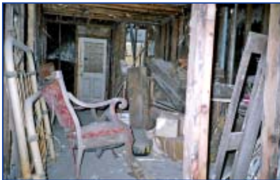
A room in a Lakeview district home after the flooding
